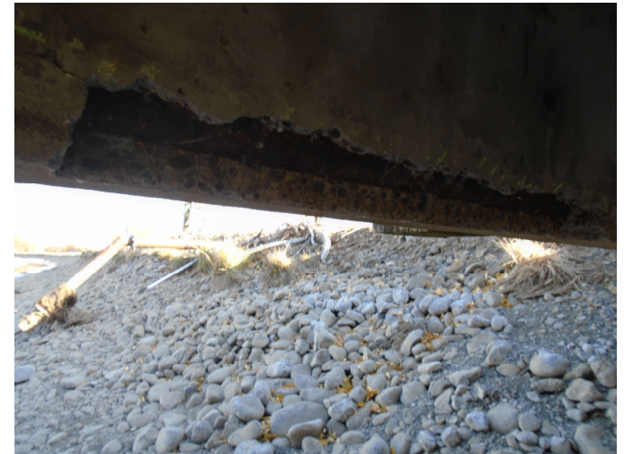
Eroding concrete girder
